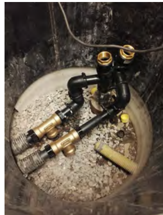
Figure 3.2: Top of the coaxial borehole
