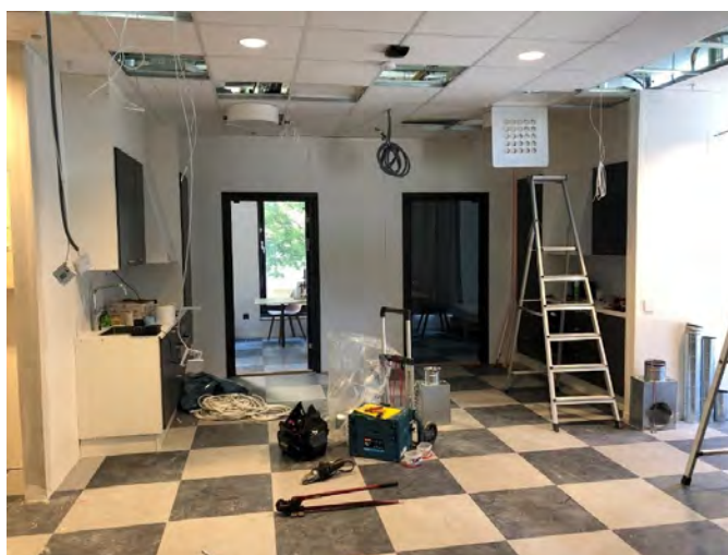
WALLS WERE REMOVED, AND SENSORS, LIGHTS AND VENTILATION WERE MOVED TO NEW POSITIONS.
