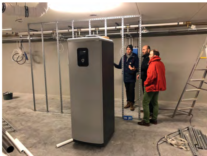
THE HEAT PUMP FROM THE RESEARCH PROJECT PARTNER, THERMIA, WHEN IT ARRIVED AT KTH LIVE-IN LAB IN 2018
