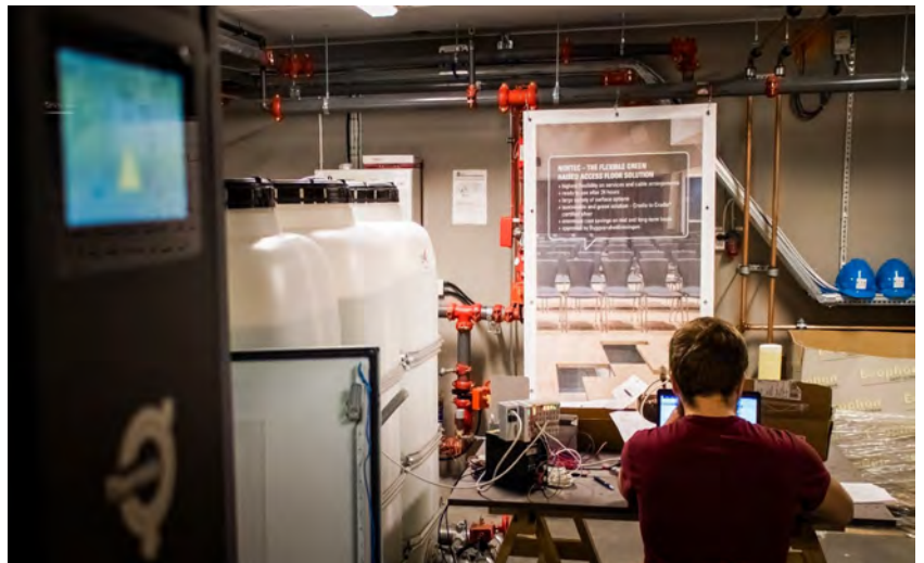
RESEARCHER ADRIEN VAUTRIN IN THE MECHANICAL ROOM OF TESTBED KTH
