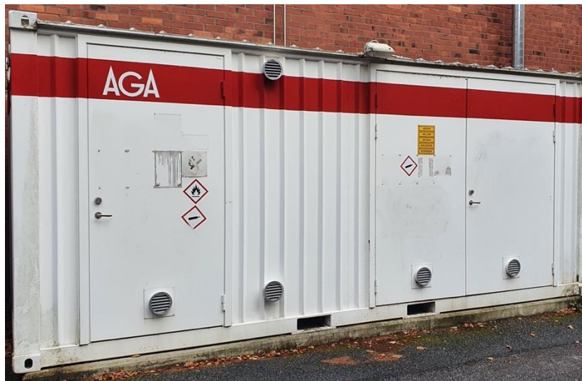
Figure 2: The gas container North.
