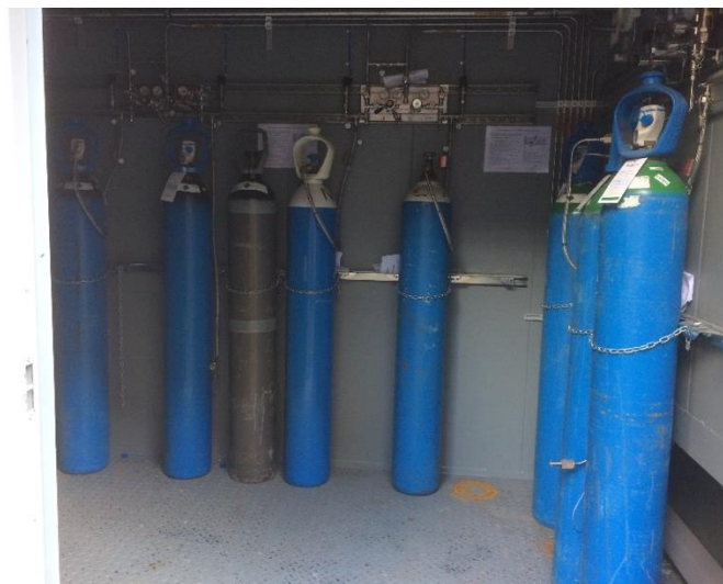
Figure 3: Inside the gas container North.
