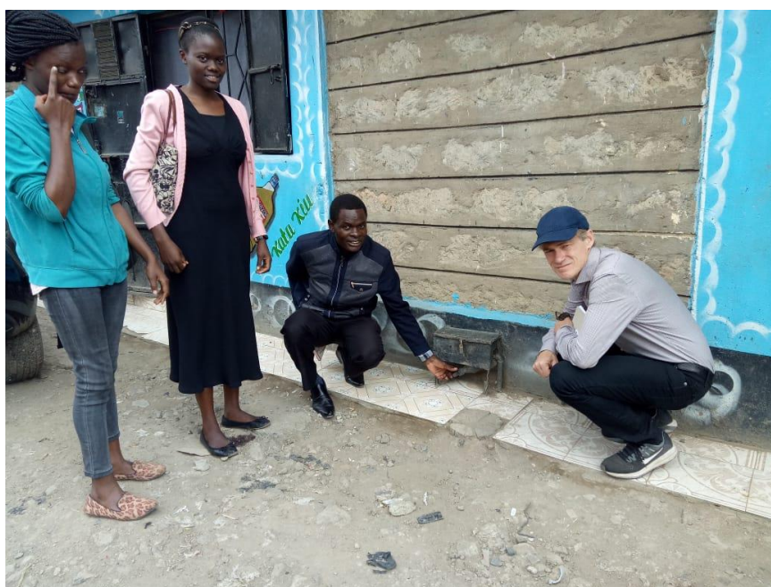
Figure 6. Self-read meter installed inside a locked meter box, in Kayole Soweto, Nairobi. Photo: Lewis Sitoki.
